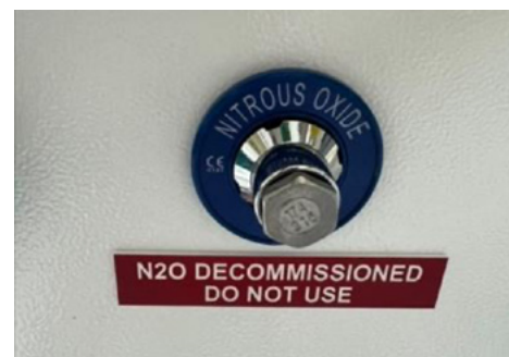
Figure 6: Decommissioned N 2 O outlet
